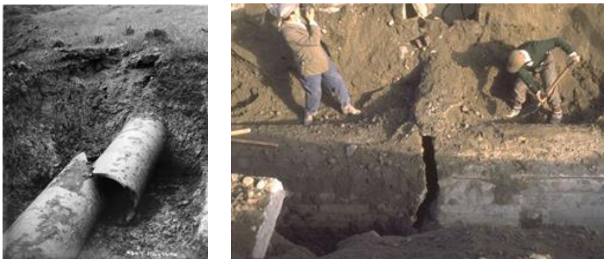
Figure 2. Appearance of pipes damaged during exploitation
