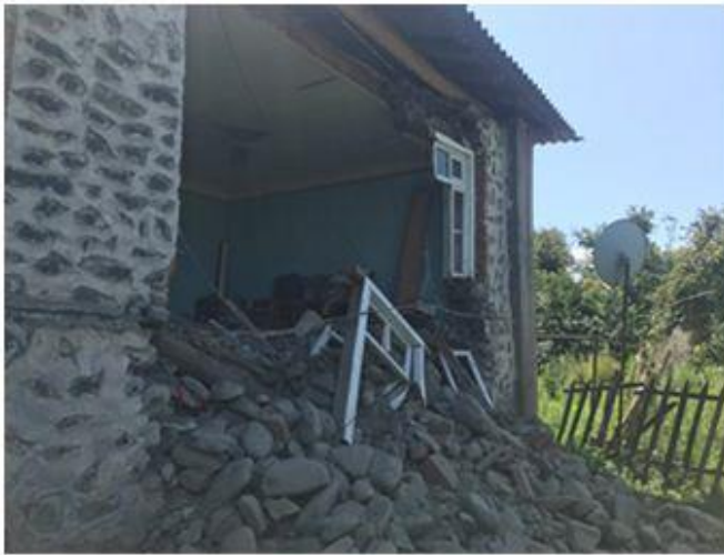
Figure 5. The collapse of the river stone wall of a house in the village of Makov
