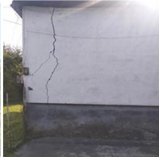
Figure 6. Old and new cracks on the wall of a house in Goyam village
