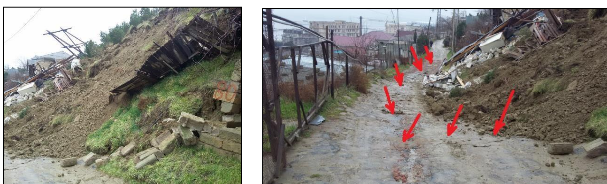
Fig. 17. Destruction, observed cracks and uplifts on the surface at a distance of 130 m from the edge of the landslide
