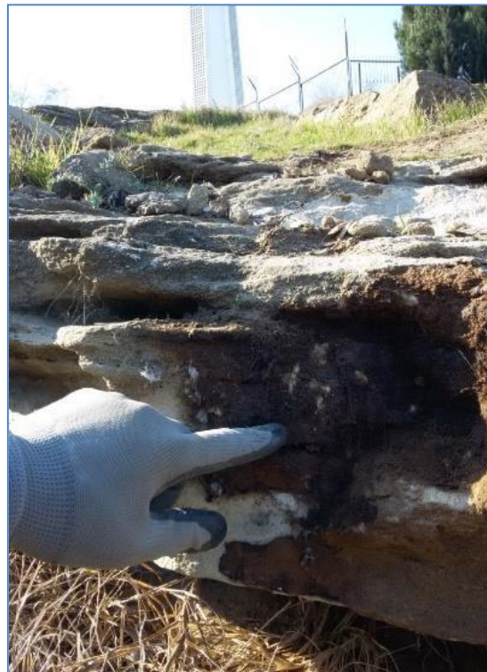
Fig. 5. Water leaks in sandstone layers in the northwestern flank of the landslide zone
